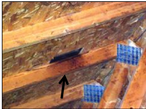
Attic III (moisture stains under cap vent)
