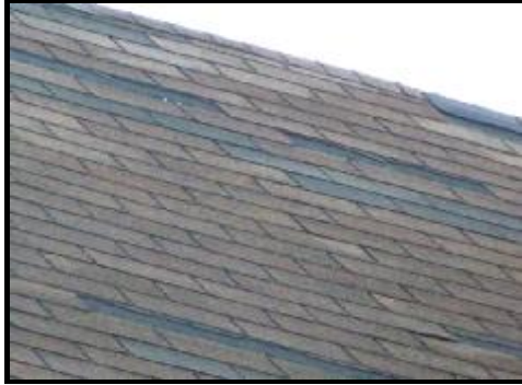
Roof IV (missing/torn shingle tabs, previous patches in front)
