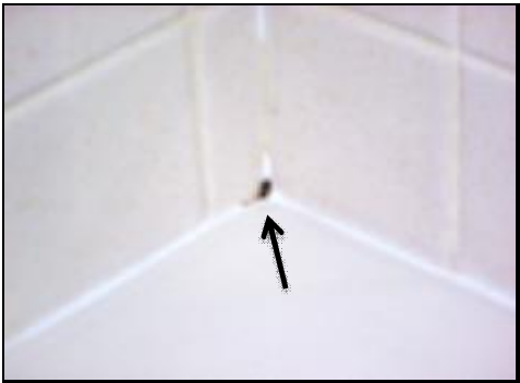
One of several open grout lines in upstairs hall bathtub
