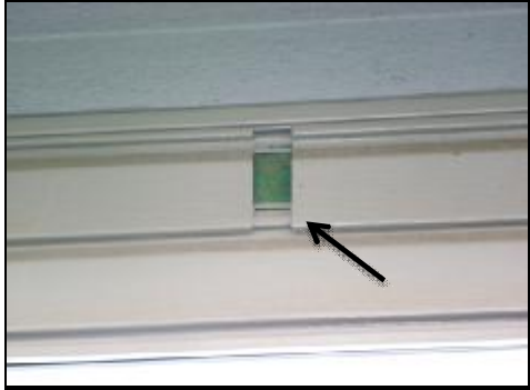
Open gap in siding (in rear)
