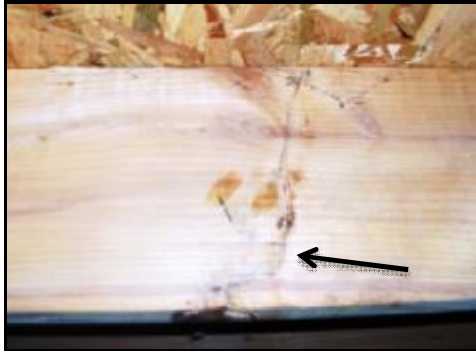
Split floor joist in crawspace (under kitchen area)
