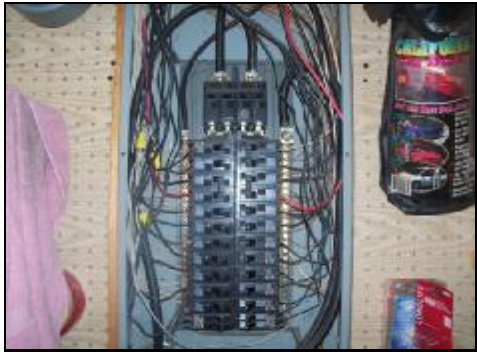
Inside main electrical panel
