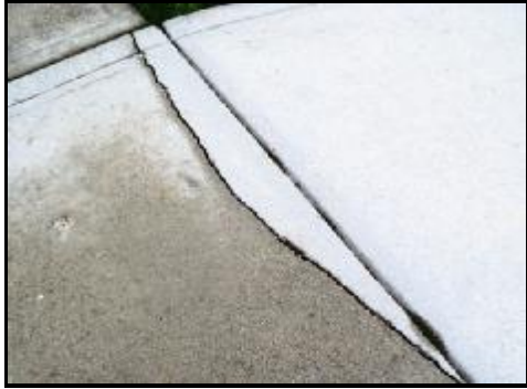
Crack on walkway
