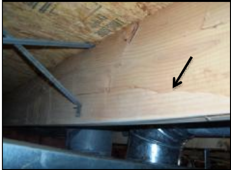
Split floor joist in crawspace (by entrance)
