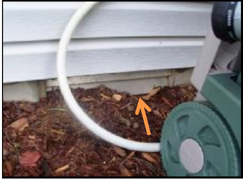
Partially covered crawlspace vent in rear
