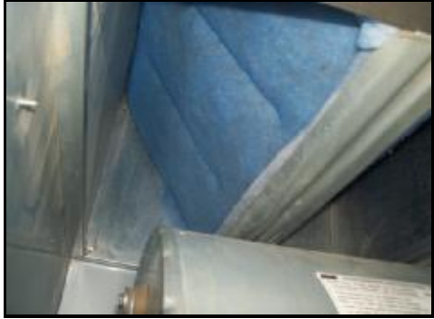
Furnace filter location
