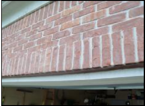
Missing weep holes on brick facing
