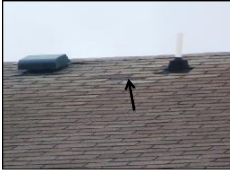
Roof V (missing shingle tab in rear)
