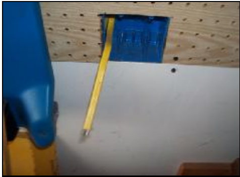
Open junction box in garage
