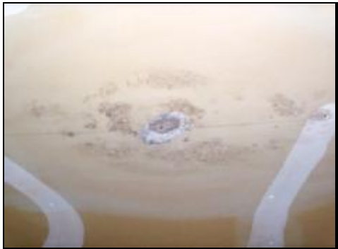
Mold stain on ceiling in 1 car garage
