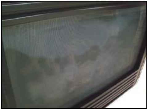
Fogged glass on direct vent gas fireplace
