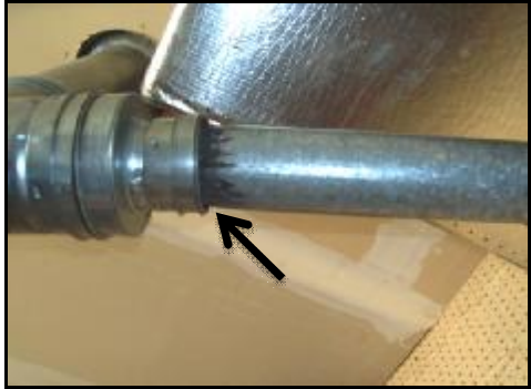
Loose water heater flue pipe connection
