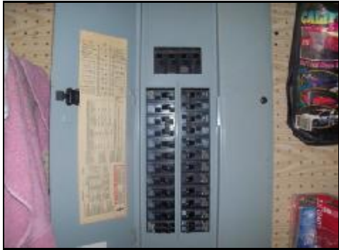
Main electrical panel
