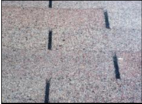
Roof III (granular loss and pitting)
