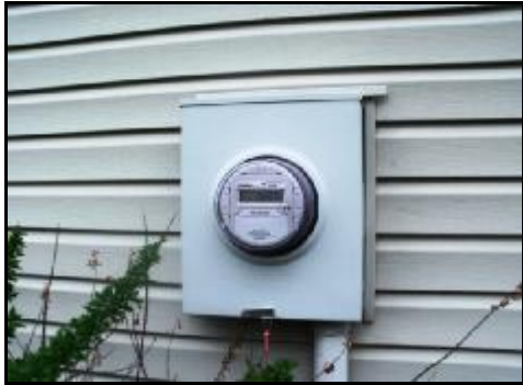
Main electrical service meter
