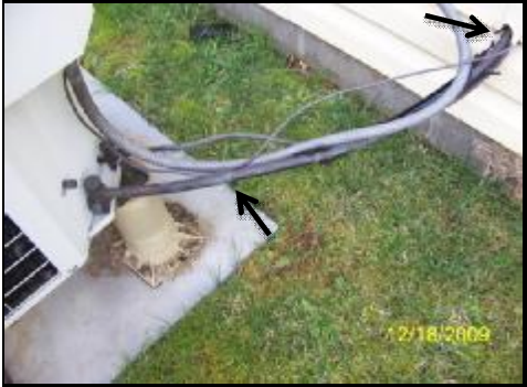
Missing insulation and HVAC putty
