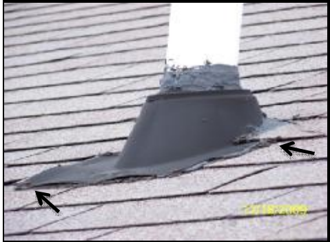
Improper installation of boot flashing and cracked sealant
