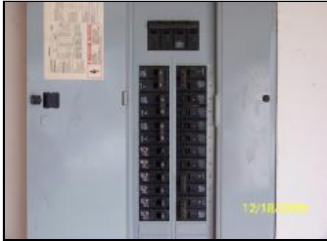
Main electrical panel
