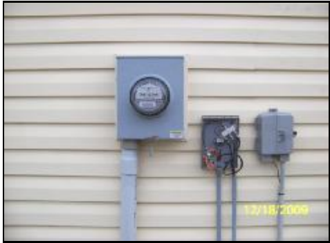
Main electrical service meter (also cable box missing cover)
