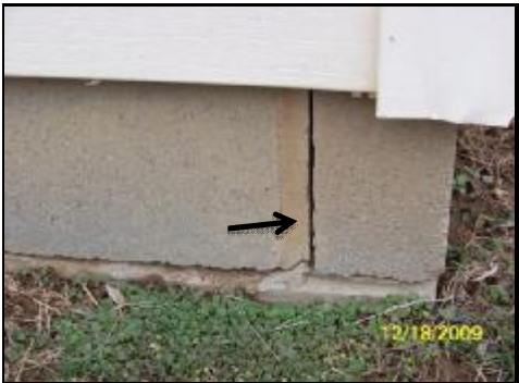
Minor tuckpointing needed II
