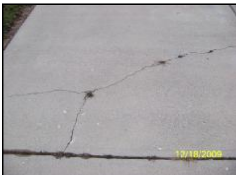
Crack in driveway
