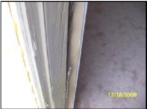
Damaged weatherstripping at back door
