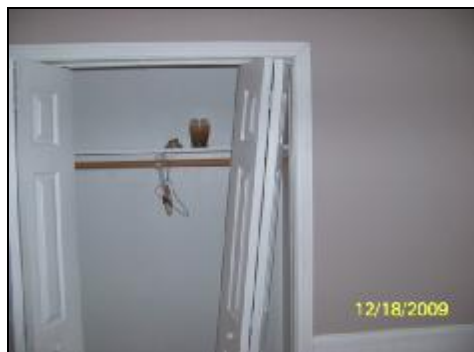
Closet door off track
