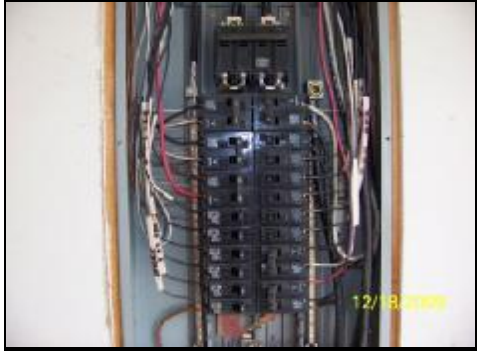
Inside main electrical panel
