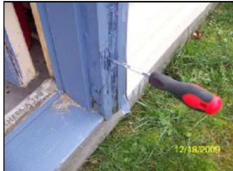
Moisture damaged moulding at side garage door
