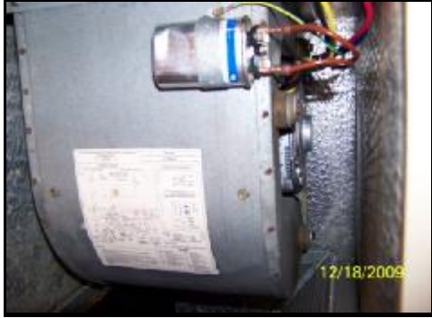
Inside furnace (blower motor)
