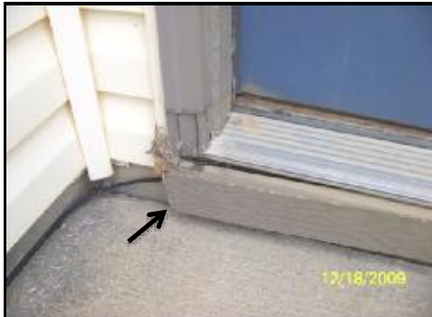
Loose trim piece at rear door
