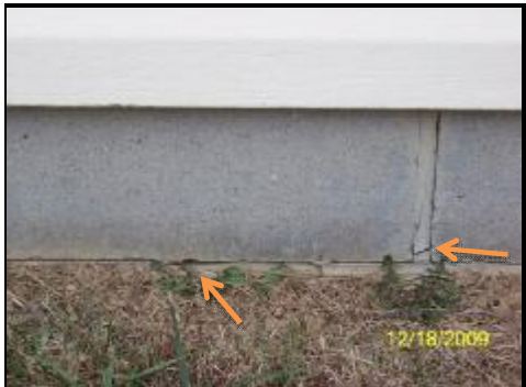
Minor tuckpointing needed
